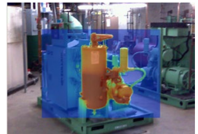
Industrial compressor, blending
